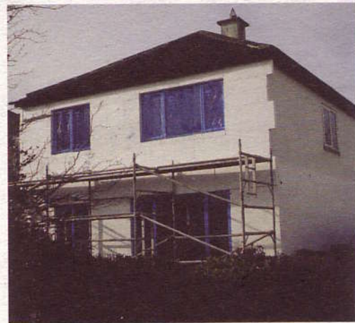
Two storey house extension and renovation by EDEN Architects which is being insulated externally
